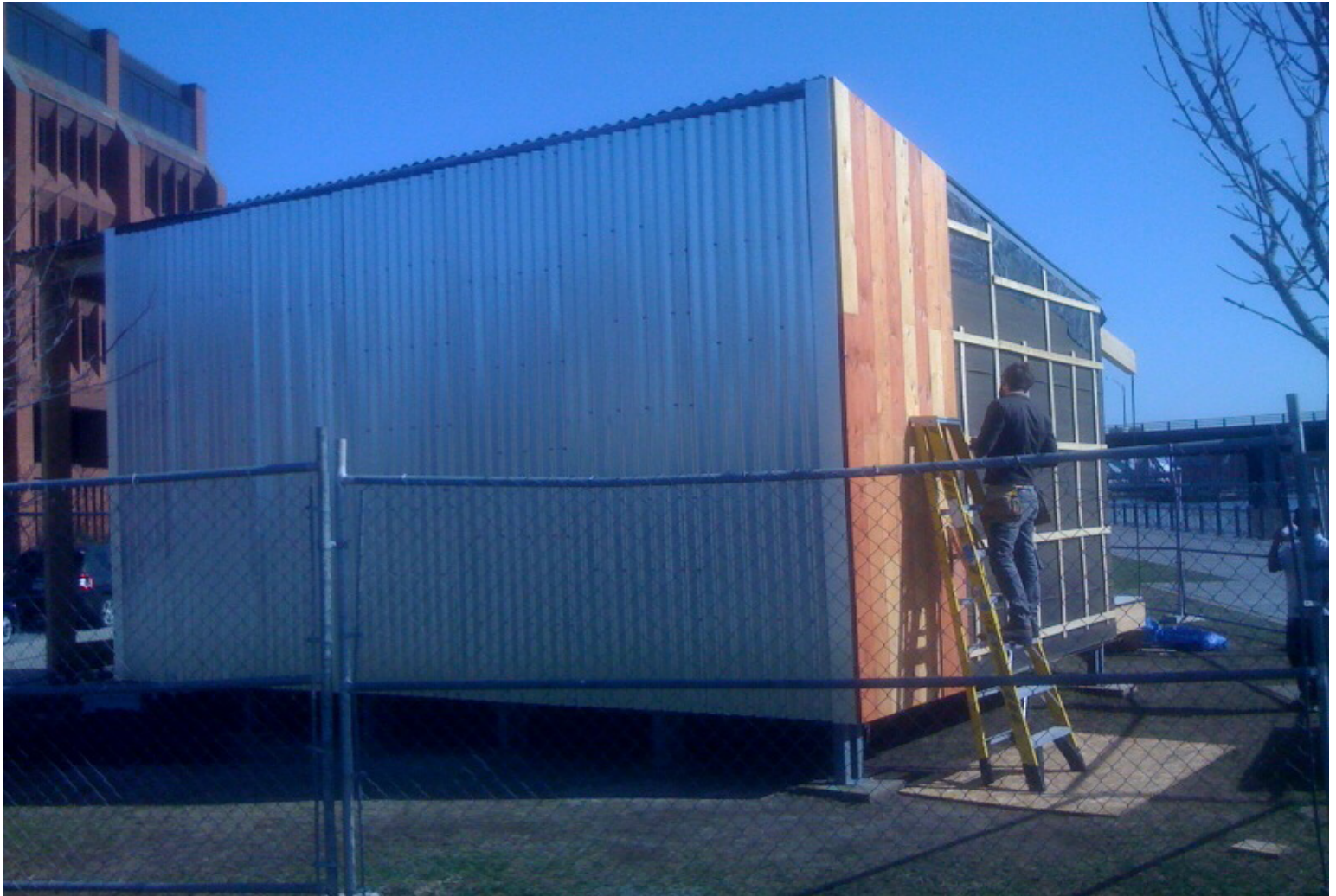
Installation of finished wood siding and corrugated metal sheathing; View looking south
